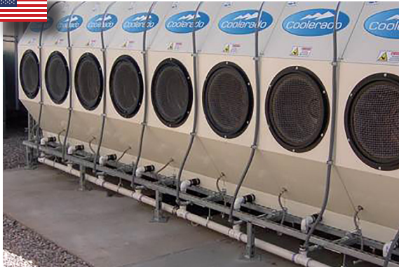
Montbello Public Library United States | Coolerado | Supplementary Cooling
