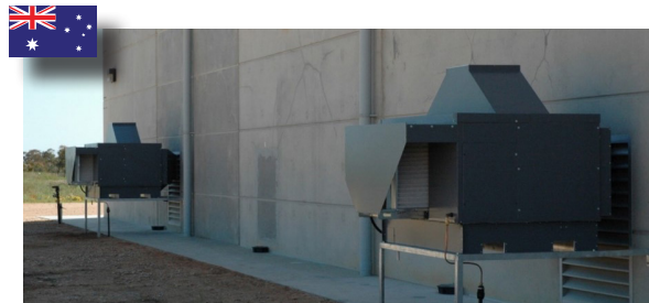
Mitolo Olive Oil Processing Plant Australia | The Climate Wizard | Stand-alone Cooling
